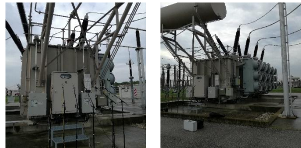
Figure 2 Transformer test site
